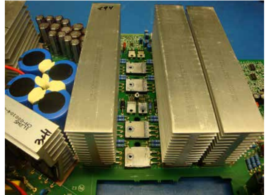
Figure 5.9 - Shorted output transistor under the heatsink (Ch2+ in this case)
