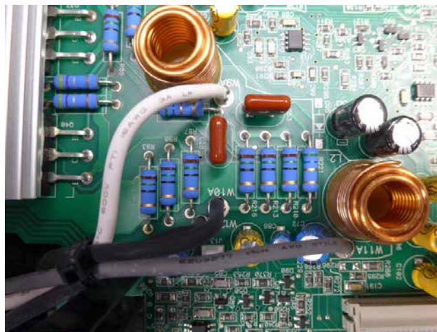
Figure 5.17 - Zobel resistors (pictured are okay) could fail due to oscillations or loose speaker wiring.
